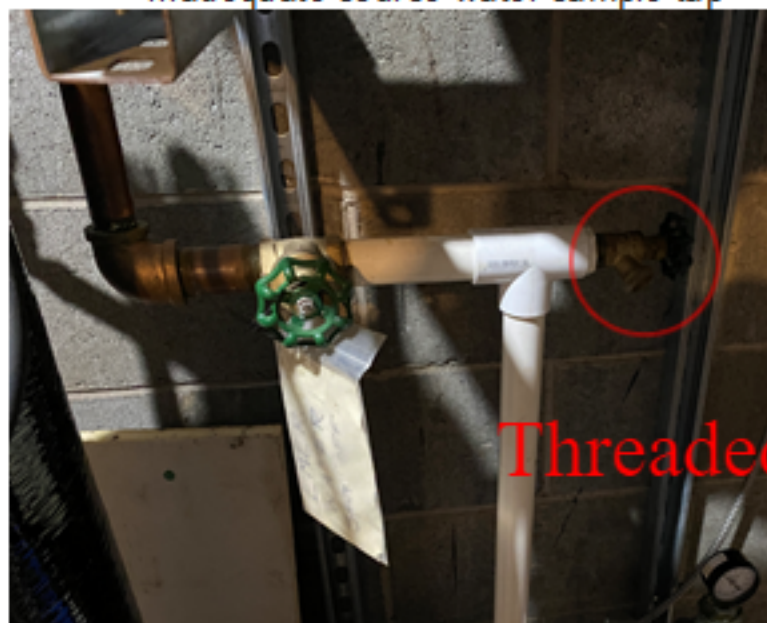
Inadequate source water sample tap
