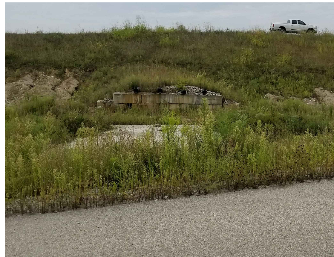
NOTE: REMOVE PIPES TO A MINIMUM 3 FEET INTO EMBANKMENT. BACKFILL VOIDS FROM DEMOLITION WITH COMPACTED SOIL FILL. MATCH ADJACENT GRADES.
