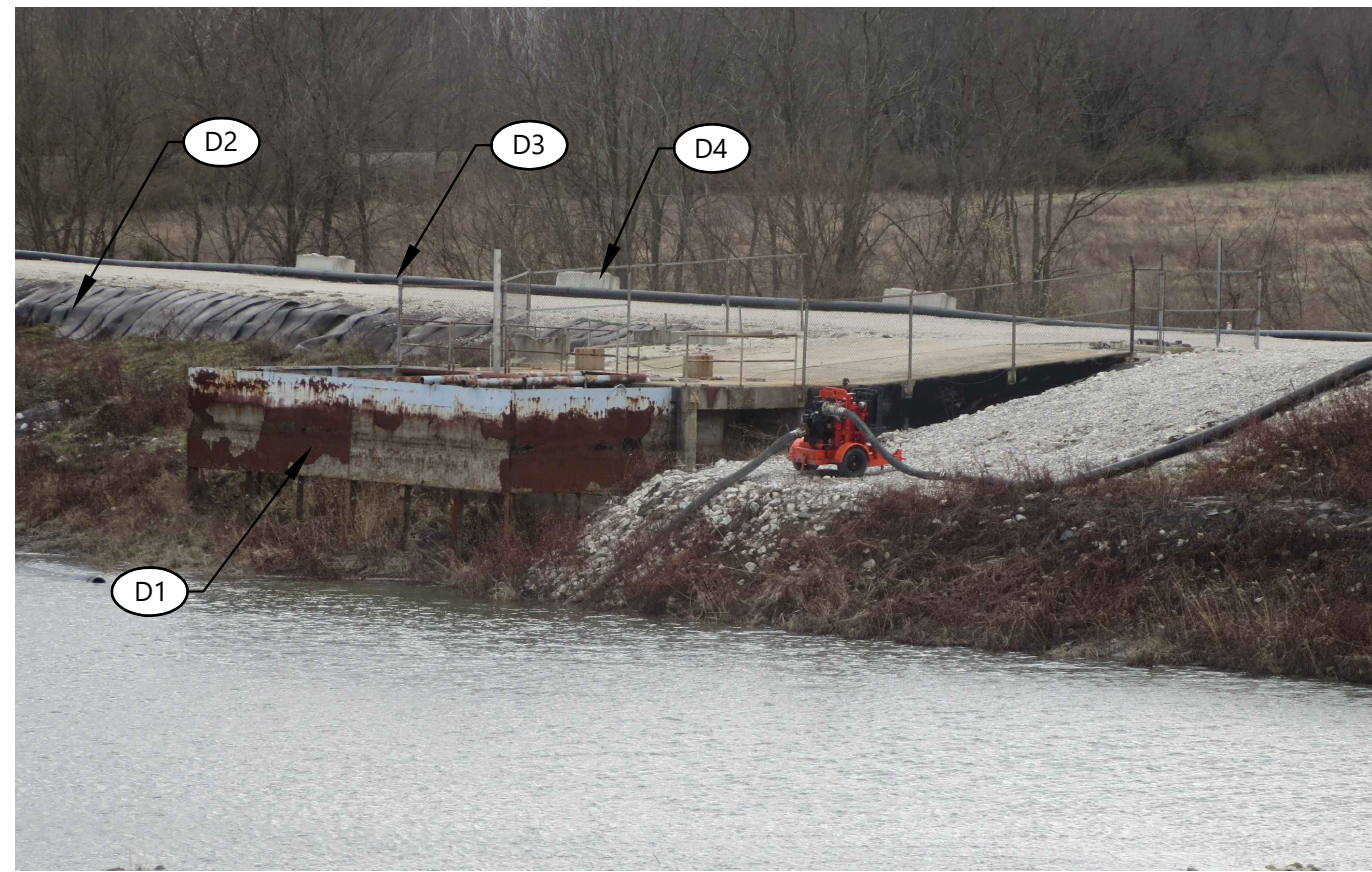
NOTE: BACKFILL VOIDS FROM DEMOLITION WITH COMPACTED SOIL FILL. MATCH ADJACENT GRADES.
