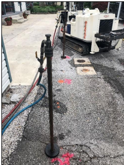
Photo 11: View looking south. Injection equipment, drill rig, and MW-9 in view. (May 21, 2020).
