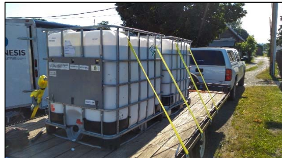
Photo 4: E – Injection trailer and product trailer staged in alley behind on-site building
