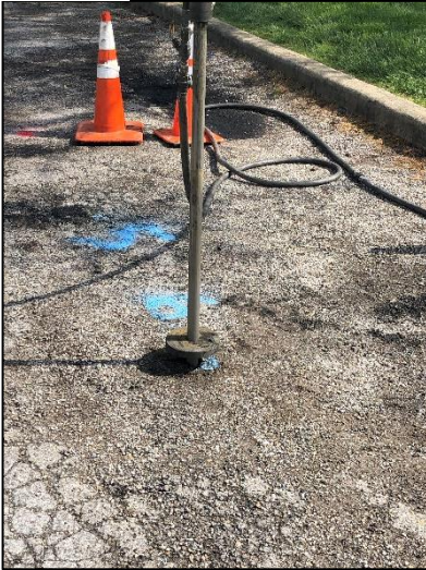
Photo 1: View looking southeast. Injection equipment and safety cones in view. (Apr 24, 2020).
