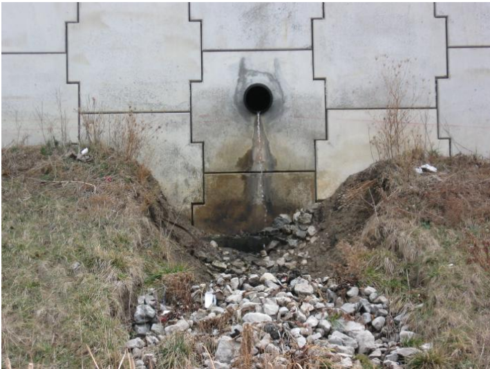
Plate 24: Storm Water Erosion from I 465
