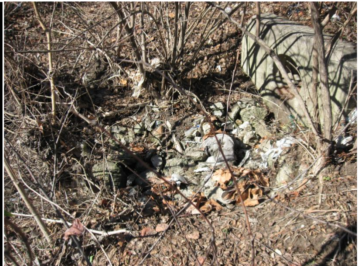
Plate 25: Storm Water Erosion from a Parking Lot Drain
