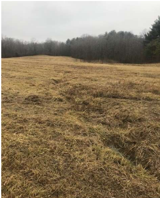
8. View to West - Vegetated/Stabilized Erosion Gully Between Terraces (To Be Repaired)
