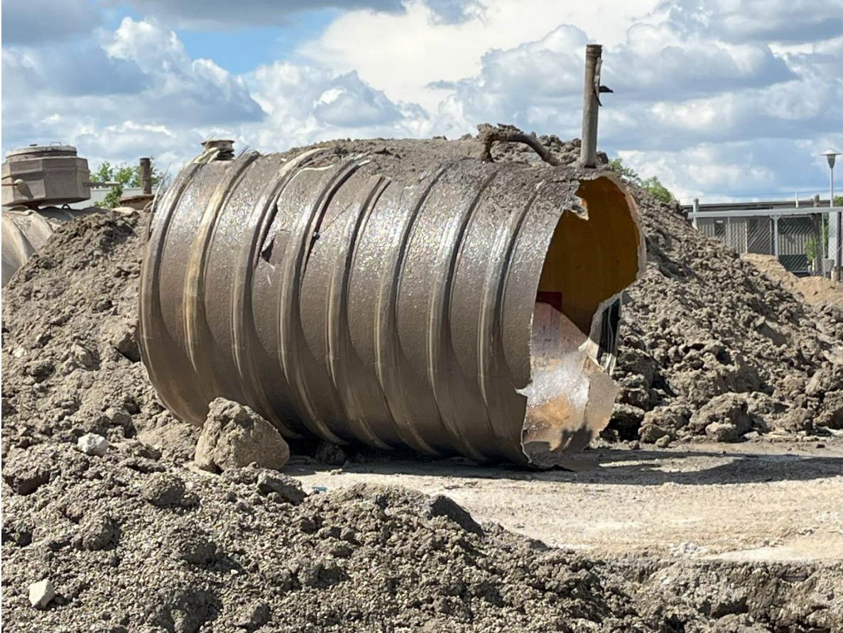
12,000 -gallon UST (brittle and collapses during removal)
