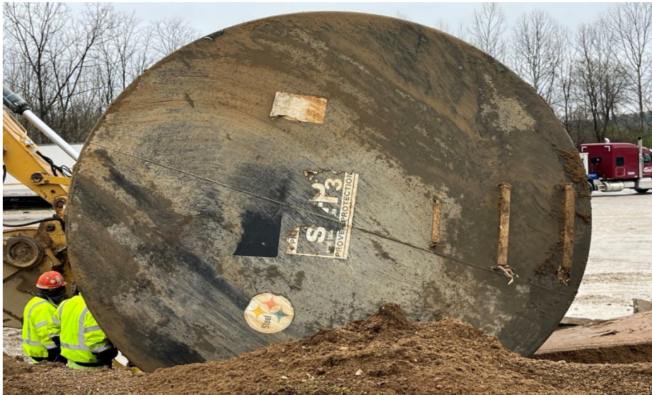
Photo 3 – Photo of the 2 nd 15,000-gallon UST from the eastern side during removal
