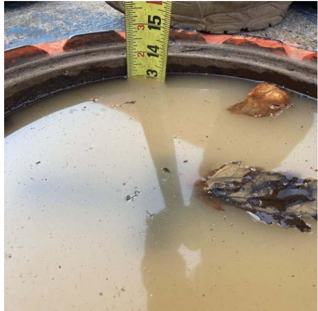
RUL VAPOR REC SPILL BUCKET TEST END 13"
