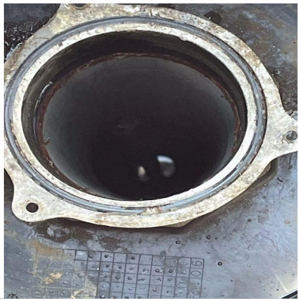
O-RING BROKEN ON RUL DROP TUBE
