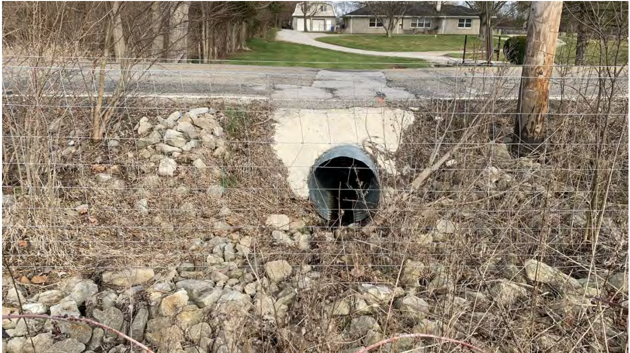
Phot 14. Looking east at the stormwater drainage outlet that Wetland K drains to.
