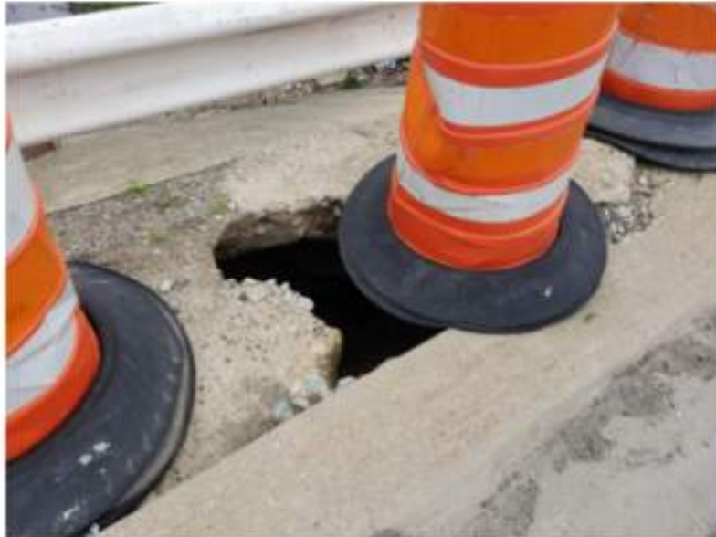
View: The concrete on the north side of the bridge over Tracy Ditch. Description: The pavement above the culvert has begun to collapse.
