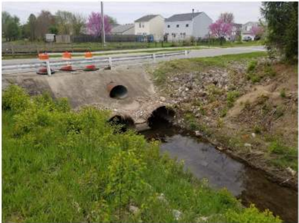
View: Tracy Ditch culvert, facing southwest. Description: The north end of the culvert over Tracy Ditch.
