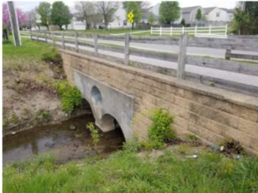
View: Tracy Ditch culvert, facing northwest. Description: The south end of the culvert over Tracy Ditch.
