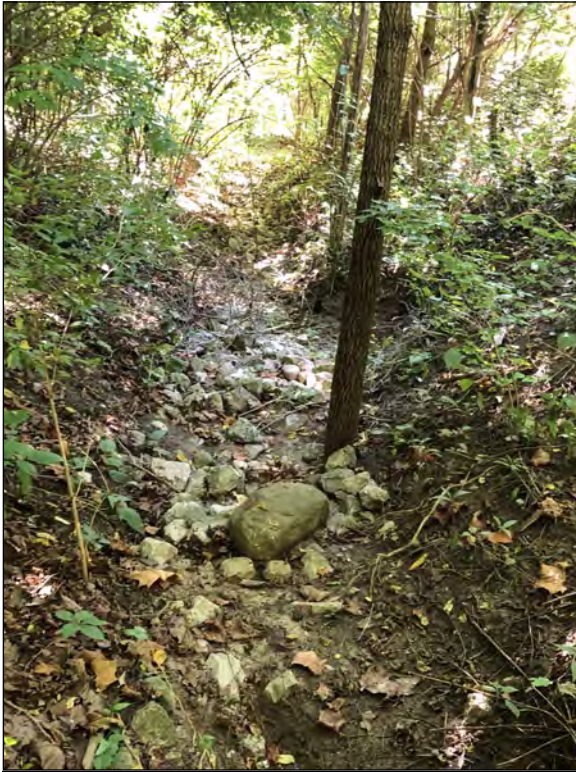
Picture 41—RSD1 riprap area—note medium-sized tree ( Juglans ) in bed; southeast view; 1 SEP 2021.
