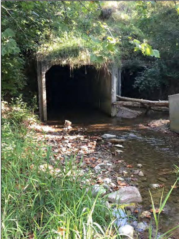
Picture 1—Goose Creek upstream and west project structure CV 026-079-28.10 , north view; 1 SEP 2021.
