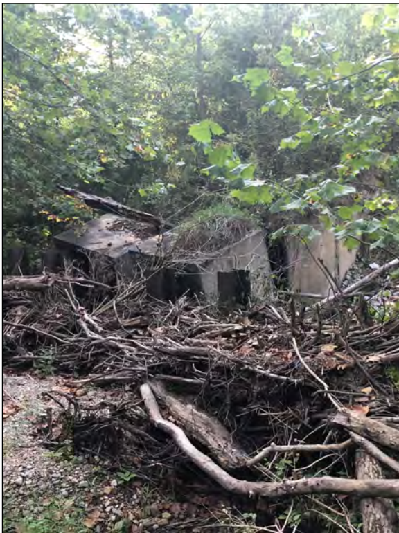
Picture 11—Goose Creek debris north of structure CV 026-079-28.10 inlet; southeast view; 14 SEP 2021. Note that steel beams have collected debris.
