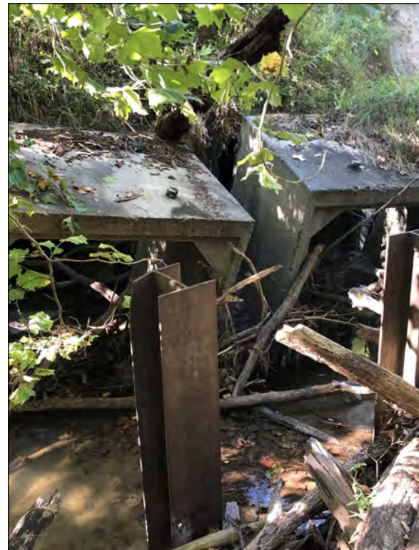
Picture 12—Goose Creek structure CV 026-079-28.10 inlet; southwest view; 1 SEP 2021. Note that culvert end pieces have detached.
