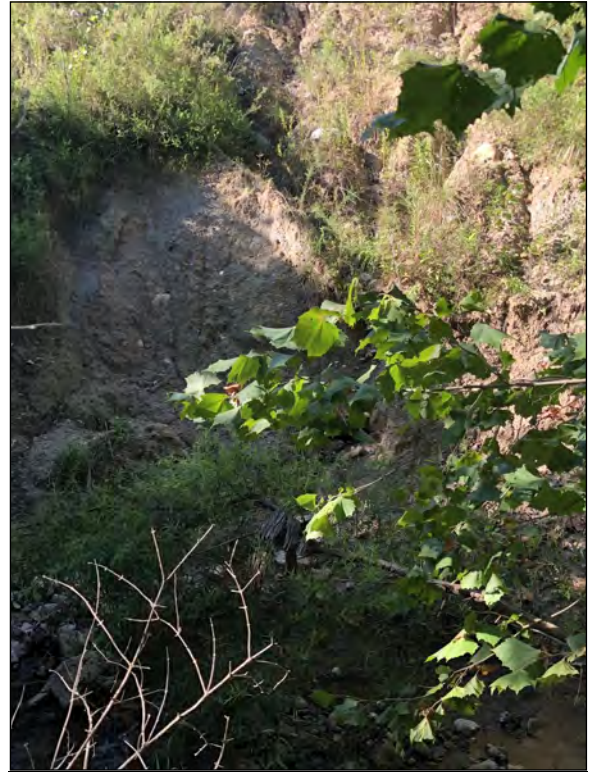
Picture 50—Eroded area west of the Goose Creek structure CV 026-079-28.10 inlet. Erosion is extensive upslope to SR 26; southwest view; 1 SEP 2021.
