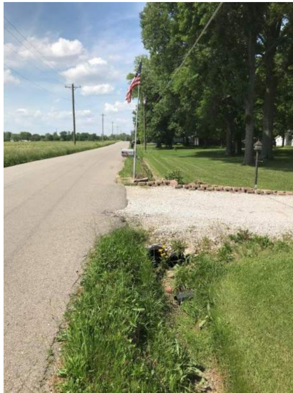
Photo 14: View of roadside culvert and dry swale along N. 850 West in Proposed Roundabout #2 (looking north).
