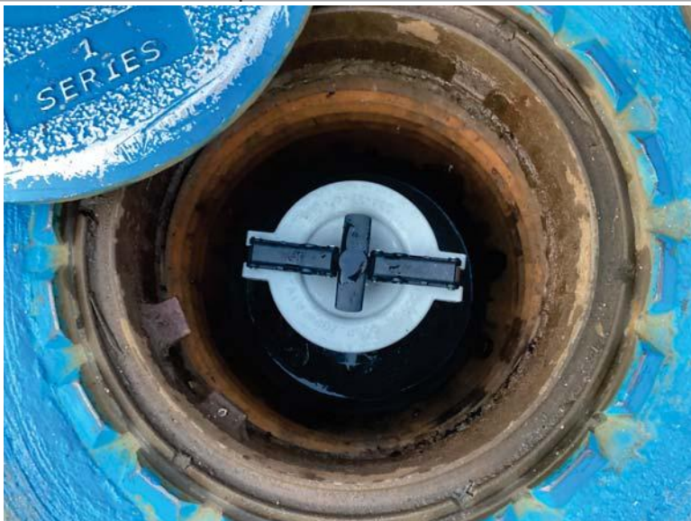
Monthly Inspection Checklist -> Spill Prevention -> Spill Containment Manhole (Spill Buckets) - Free of water and product
