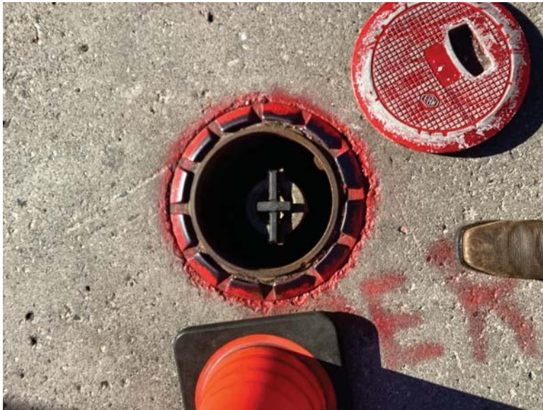
Monthly Inspection Checklist -> Spill Prevention -> Spill Containment Manhole (Spill Buckets) - Free of water and product
