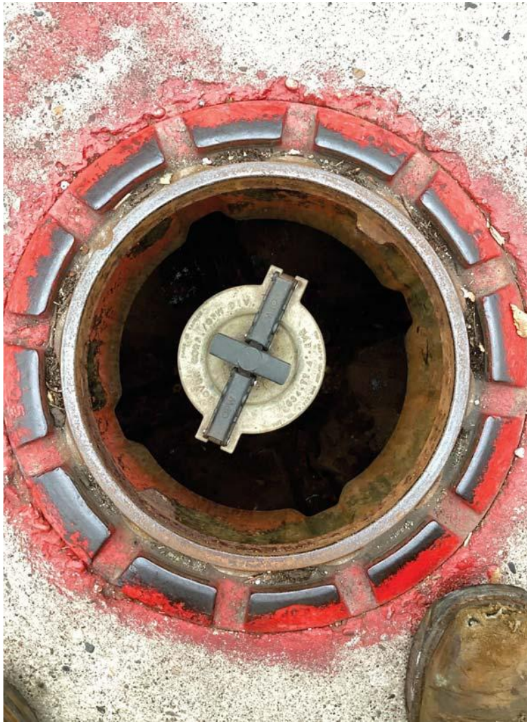
Monthly Inspection Checklist -> Spill Prevention -> Spill Containment Manhole (Spill Buckets) - Free of water and product
