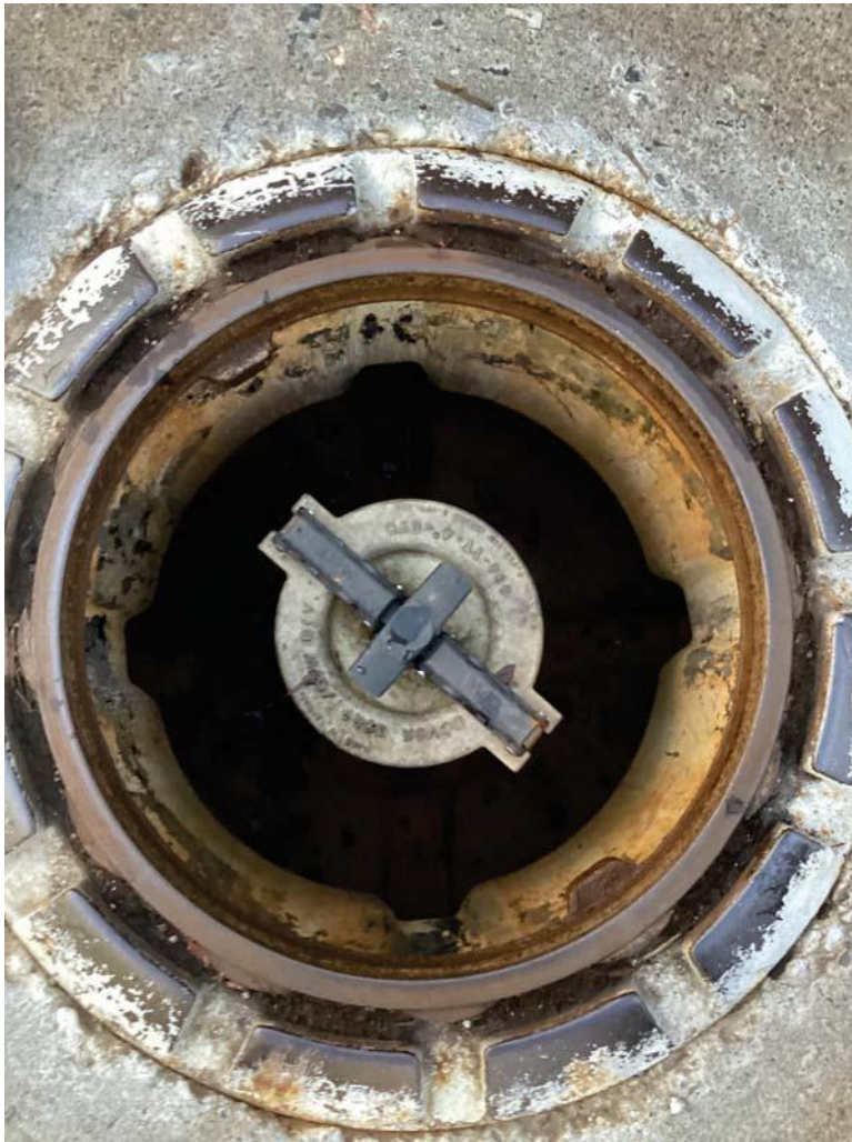
Monthly Inspection Checklist -> Spill Prevention -> Spill Containment Manhole (Spill Buckets) - Free of water and product
