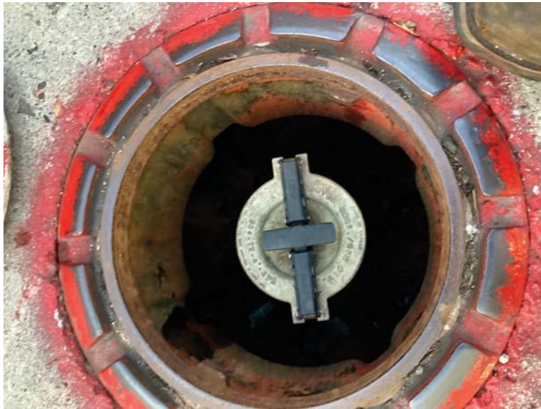
Monthly Inspection Checklist -> Spill Prevention -> Spill Containment Manhole (Spill Buckets) - Free of water and product
