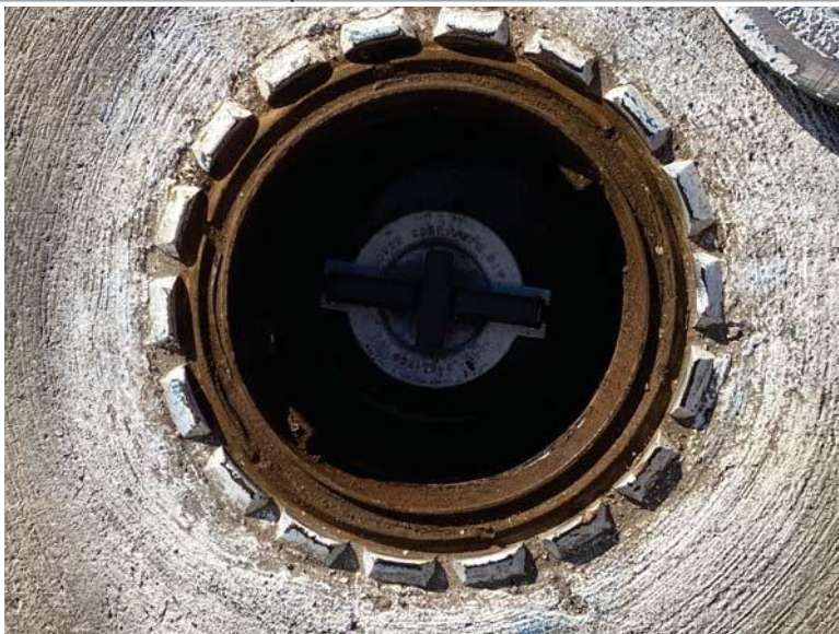
Monthly Inspection Checklist -> Spill Prevention -> Spill Containment Manhole (Spill Buckets) - Free of water and product
