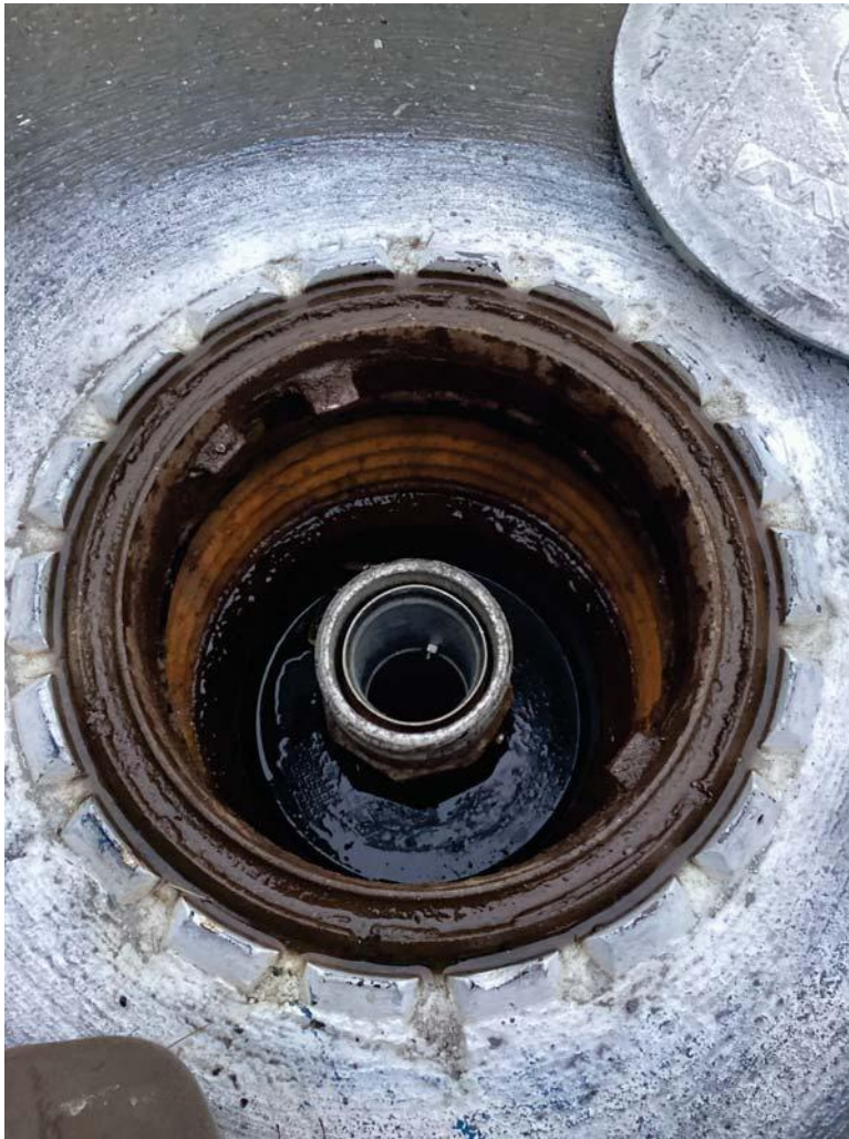
Monthly Inspection Checklist -> Spill Prevention -> Spill Containment Manhole (Spill Buckets) - Free of water and product
