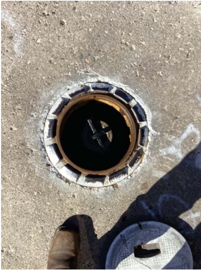
Monthly Inspection Checklist -> Spill Prevention -> Spill Containment Manhole (Spill Buckets) - Free of water and product
