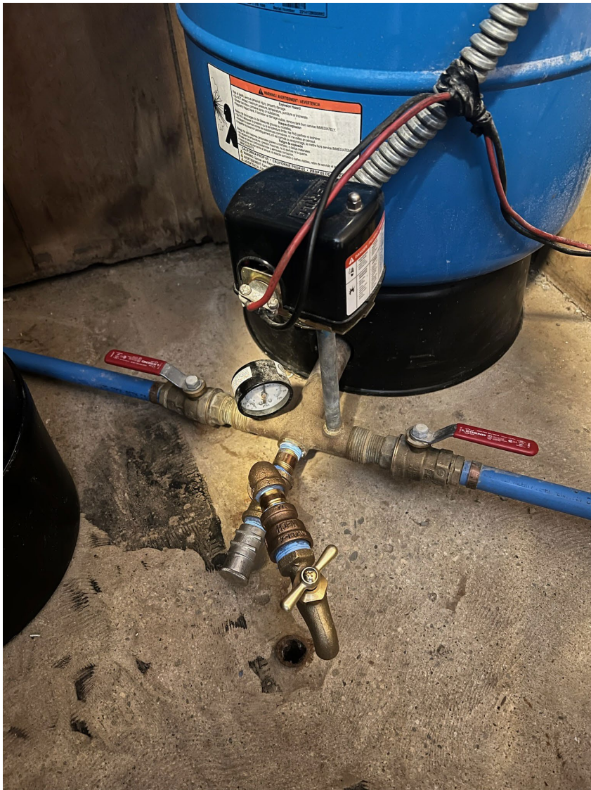
A vacuum breaker has been installed on the outside spigot as requested.
