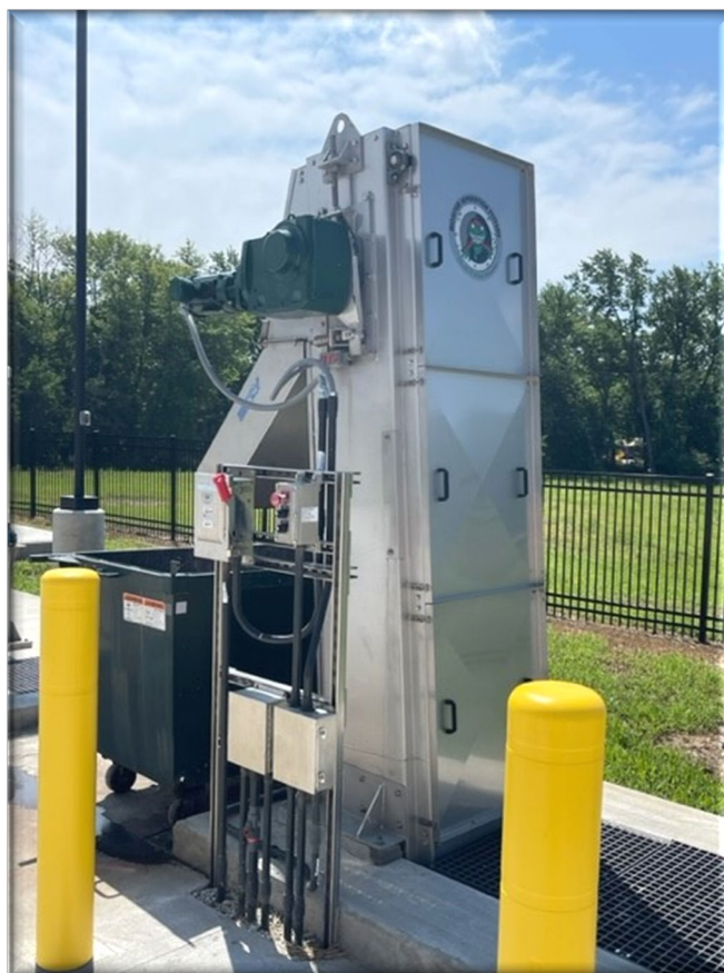
Photograph 6-4 – Muffin Monster Vertical Bar Screen at New Main Lift Station
