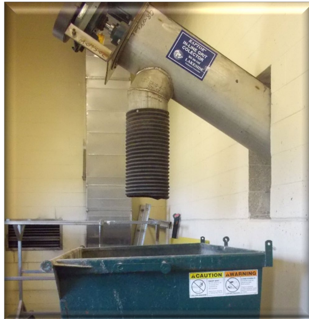
Photograph 6-1 – Raptor In-Line Grit Collector
