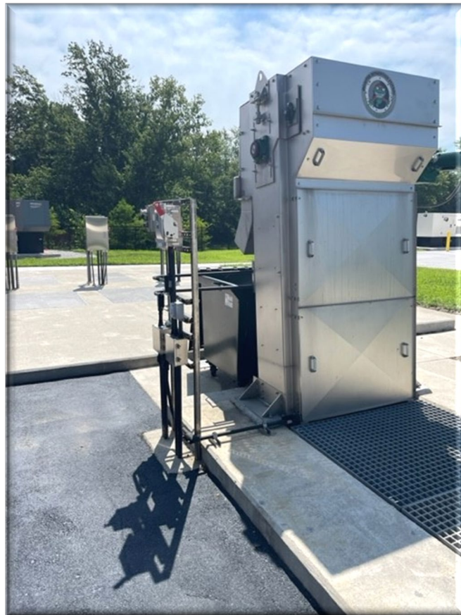
Photograph 6-3 – Muffin Monster Vertical Bar Screen at Wet Weather Treatment Facility
