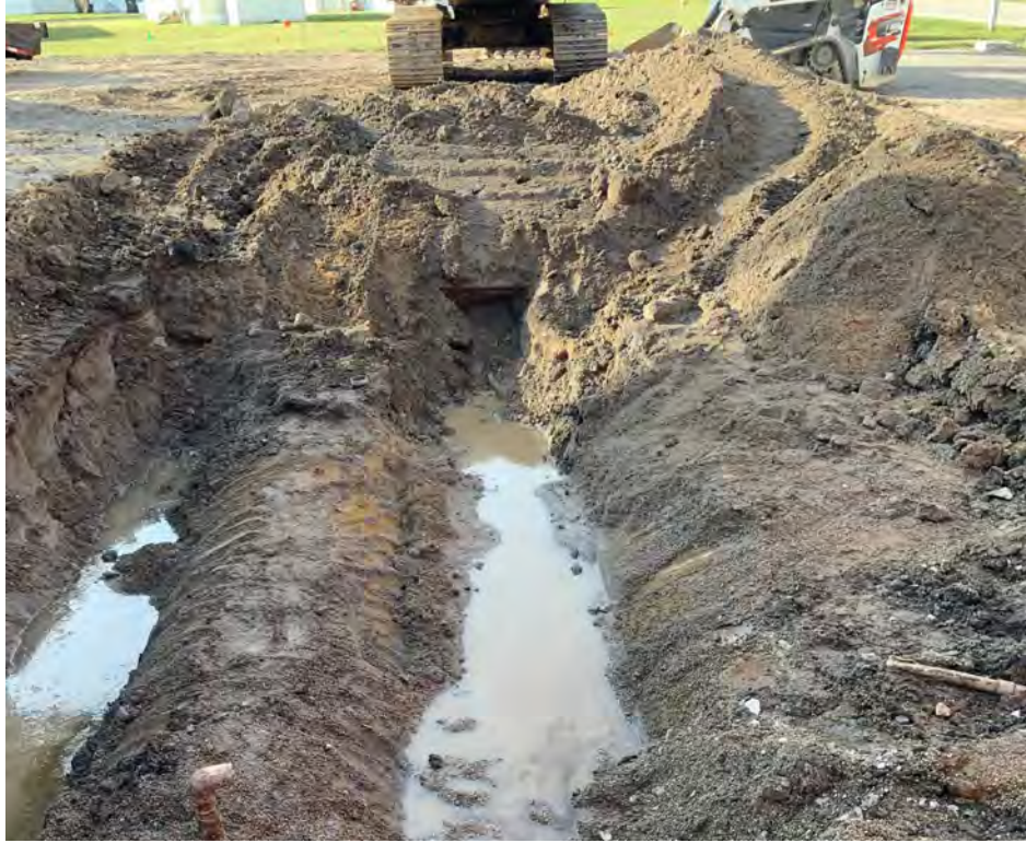
Photo 1: Diesel tank basin. Diesel tank exposed and orphan tank discovered..
