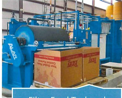
Filter Feed Tank and Dewatering Filter Skid
