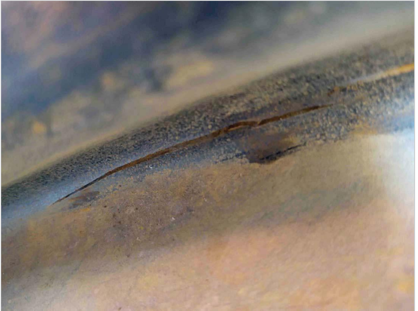
RUL fill SW EBW SB failed due to crack on side wall.
