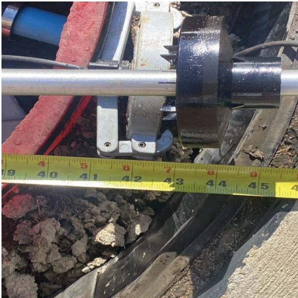
DSL EAST ATG PROBE TEST
