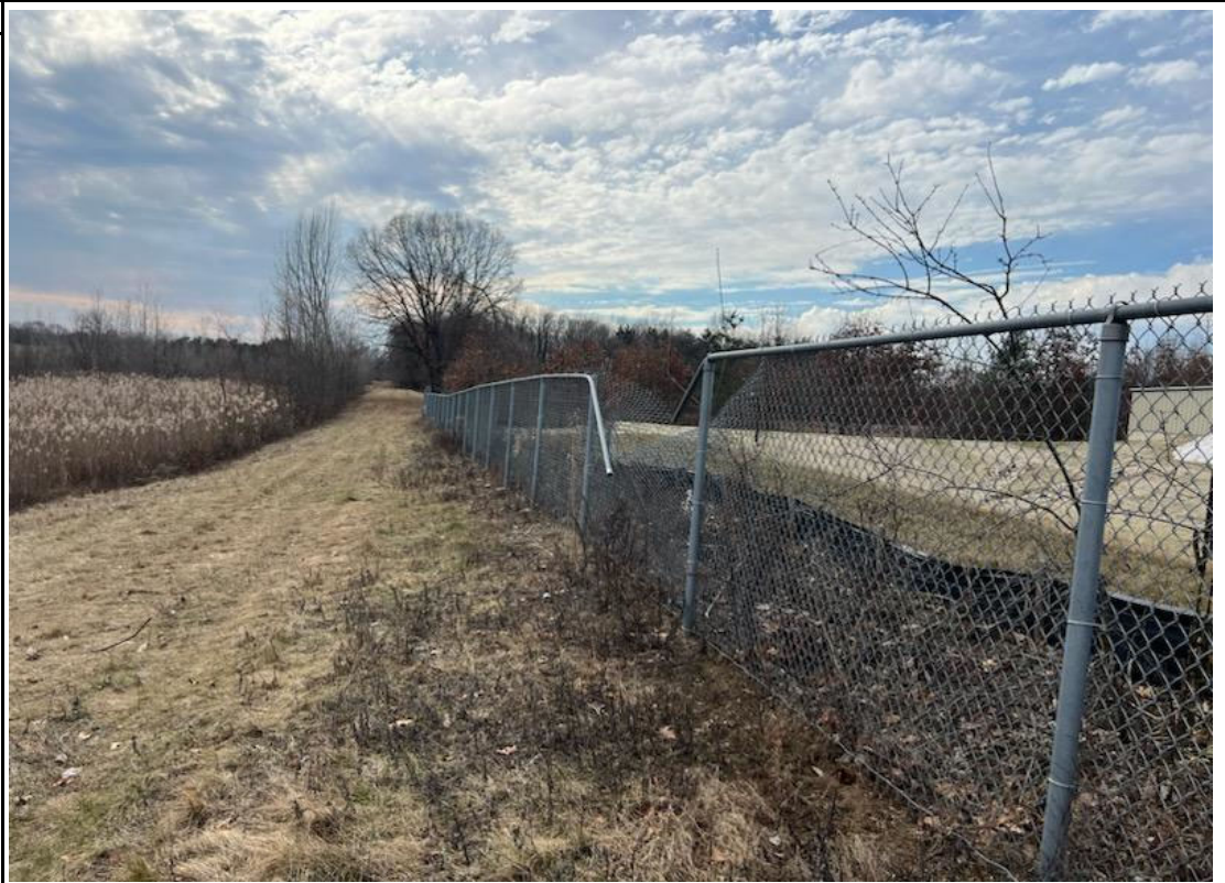
Photo #3 View of damaged fence on western property boundary.
