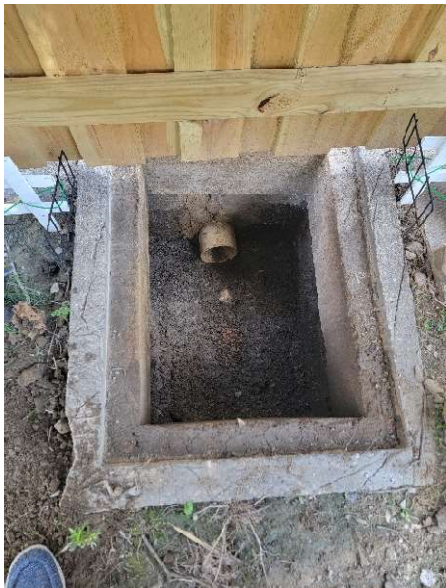
View of inside of exterior vault.
