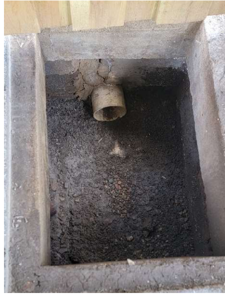
View of 4-inch pipe leading to the east toward the sanitary sewer.
