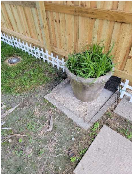
Flowerpot on top of exterior vault located near the southeast corner of site building.
