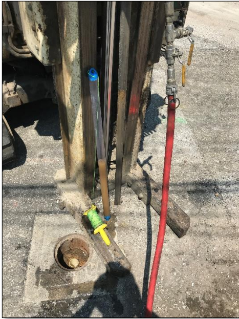
Photo 5: View looking north. GeoProbe drill rig in view while injecting on IP-19. Bailer showing no influence on MW-10 prior to injection. (August 2, 2018)
