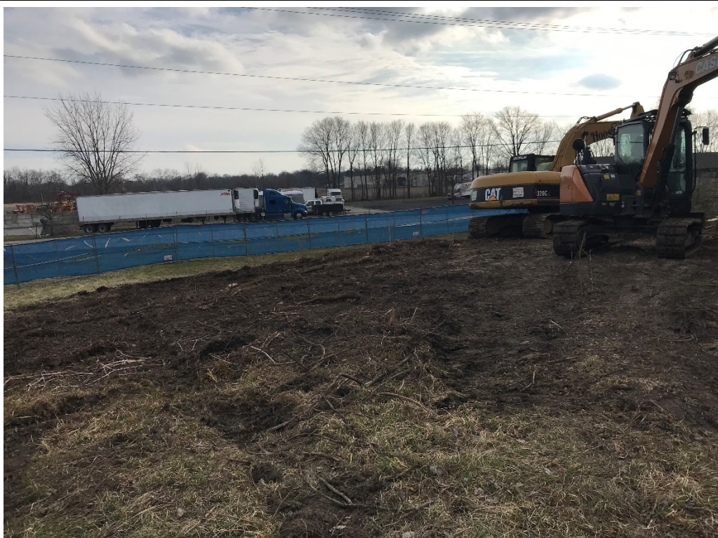
Photo 2: Excavation area cleared of trees; fencing to enclose work area in place (February 11)
