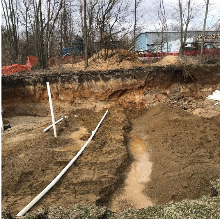
Photo 11: Trench into groundwater for Injection Line 3; Injection Line 2 on the left (February 20)
