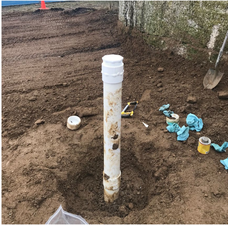
Photo 21: New adaptor placed on Injection Lines to connect to injection hose (March 3)
