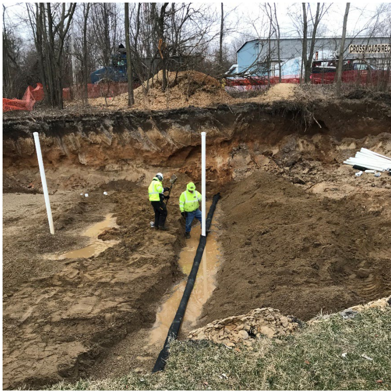
Photo 12: Placement of Injection Line 3 on pea gravel waiting for additional gravel (February 20)
