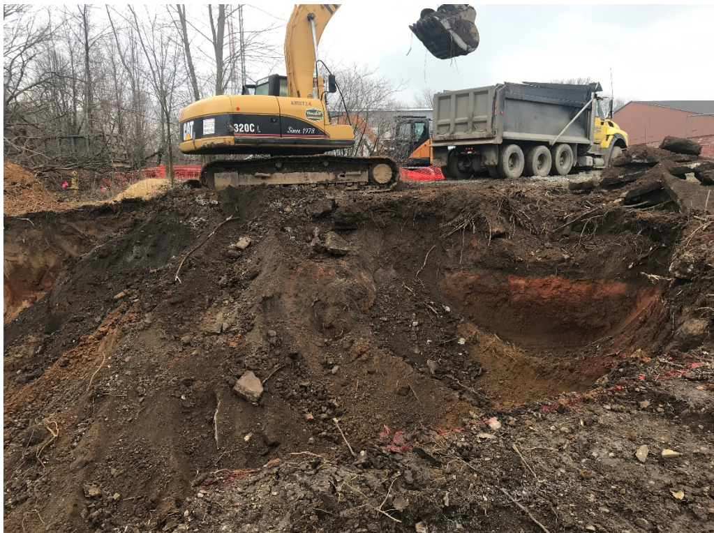
Photo 7: Excavator loading into dump truck; clay layer and debris observed in NE corner of excavation area (February 18)
