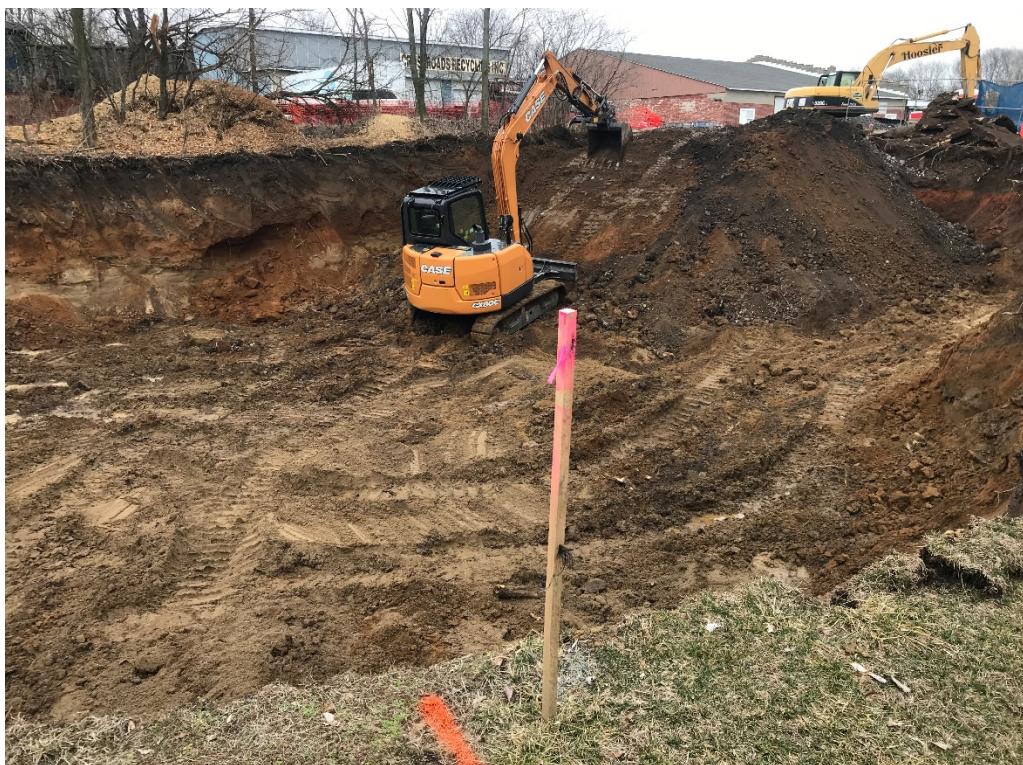
Photo 8: Remaining soil to be excavated in NE corner of excavation area (February 18)
