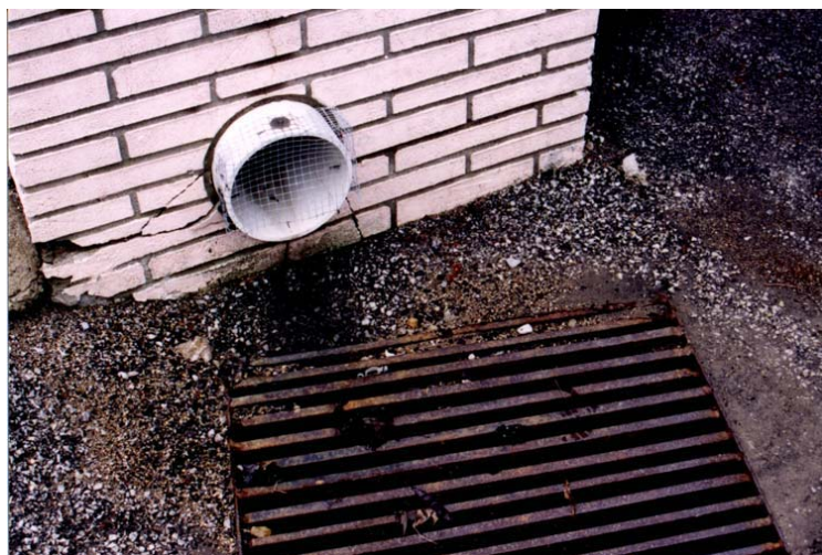
Figure 55. Sample Storm Drain Infrastructure
