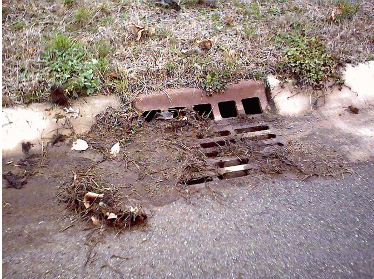
Figure 58. Typical Street Drain to Lake Tippecanoe
